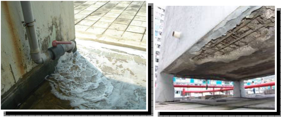
Fig. 3 Water Ponding and Damages to Roof Structure
