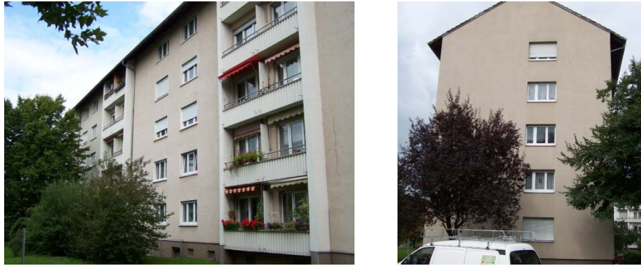
Figure 2 West façade (left picture) and south façade (right picture) of the first block, before refurbishment
