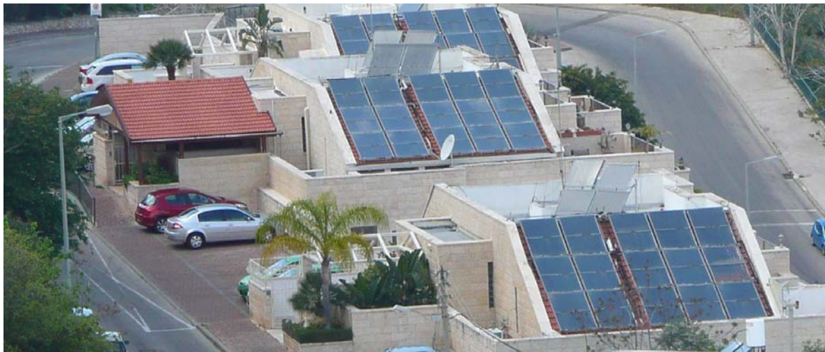
Fig. 3. Solar collectors for Hot Water
