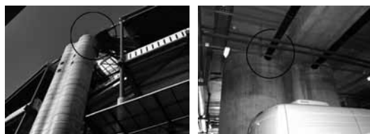
Fig.8 and 9: Details of entry and exit system of the pillars of the "Estádio da Luz"
