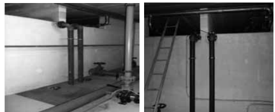
Fig.12 and 13: 3 deposits in the basement of the "Estádio da Luz"
