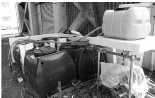
Fig. 2 – Water Storage Tank (left) and Rainwater receiving tank (right)
