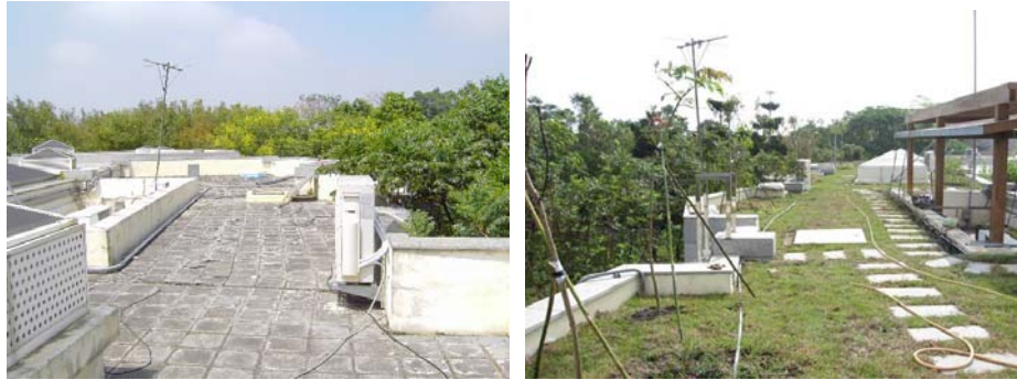
Figure 11 Before (left) and after (right) creating a rooftop garden in the service center of Tai-chung Metropolitan Park (source: ABRI, 2008)
