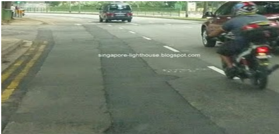
Figure 3. Uneven Road Surfaces
