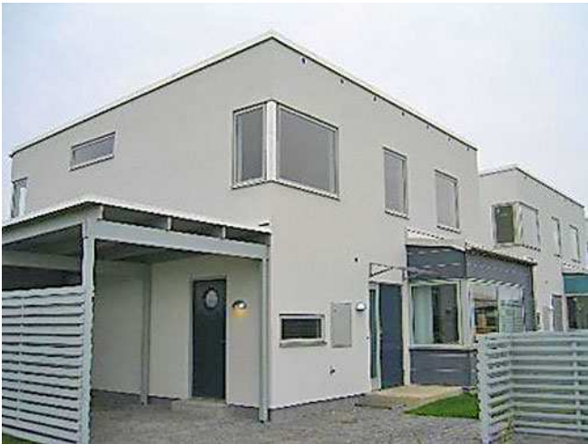
Fig 2.2 Stucco facades with problem
