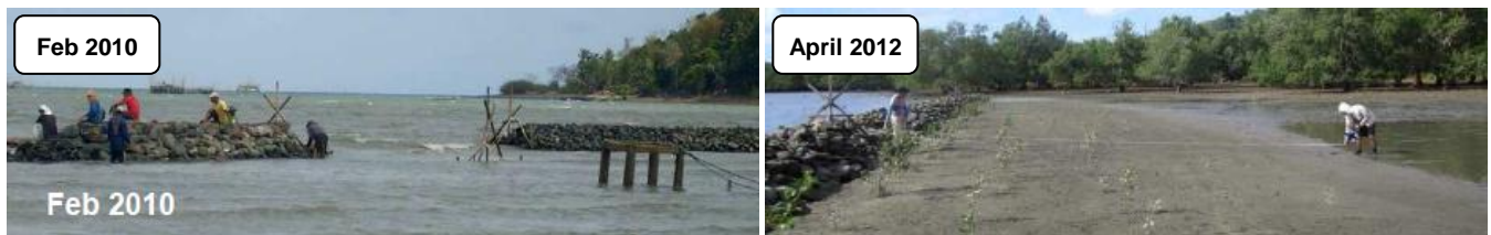
Figure 12 (left) Breakwaters completed in 2010; (right) accreted sediments after 26 months, mangrove saplings transplanted, and fully grown mangroves seen in the background (ZSL-CMRP photos by J.H. Primavera (left) and A.M. Torrechilla)
