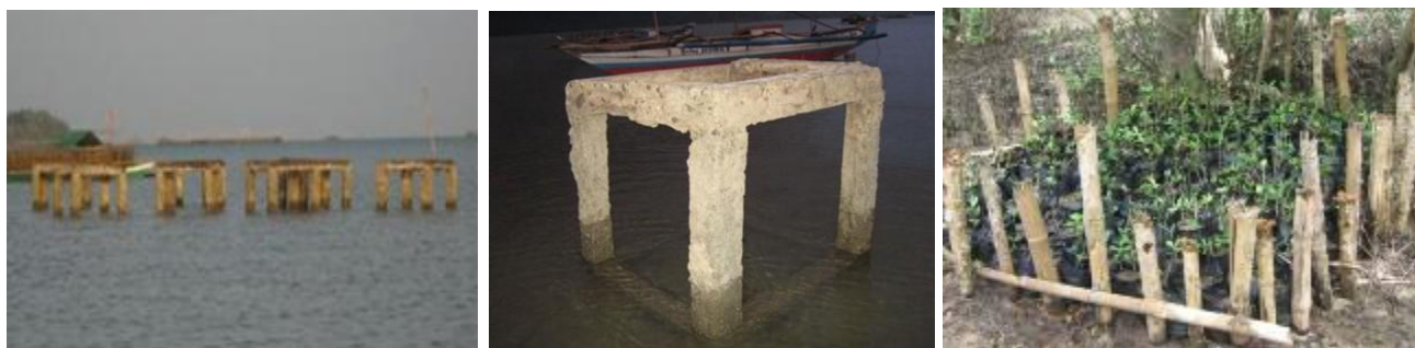
Figure 3 (left) Damaged “modules”; (middle) closer view of a module; (right) mangrove seedlings in inland nursery
