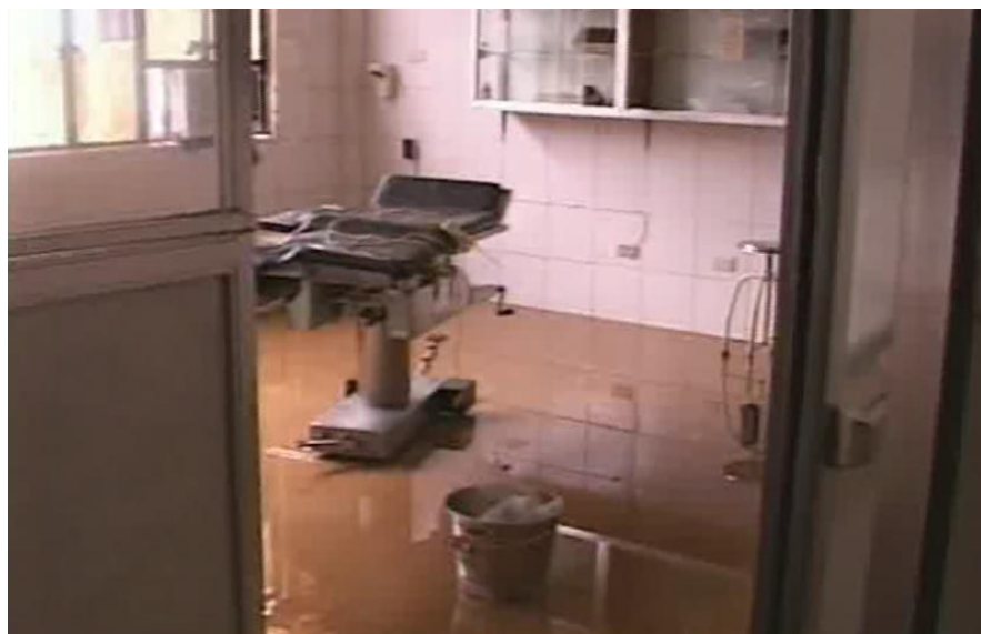
Figure 2 Emergency Room of DRSTMH in Aklan (Source: Screen Capture from DOH Video)
