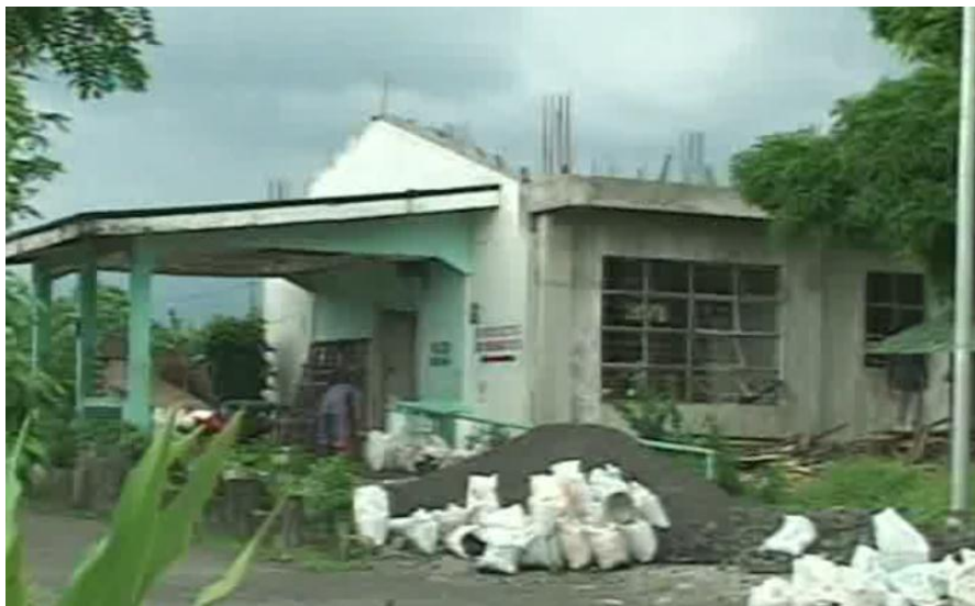
Figure 3. JBDMDH in Ligao City without a roof because of Typhoon Reming and Milenyo (Source: Screen Capture from DOH Video)
