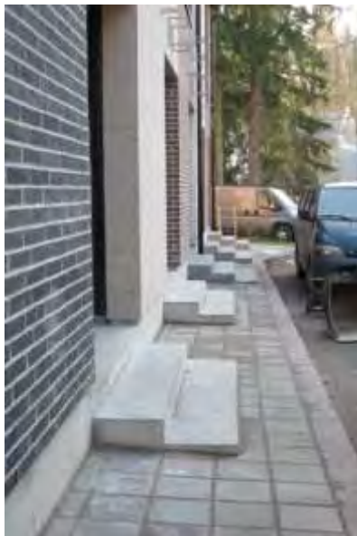
Fig.7. Newly built townhouses (2014) directly attached to the street with on street parking. Due to incompatibility of building and street realization the building does not fulfill requirement for accessibility or visitability. (Ormuspelto, Helsinki).
