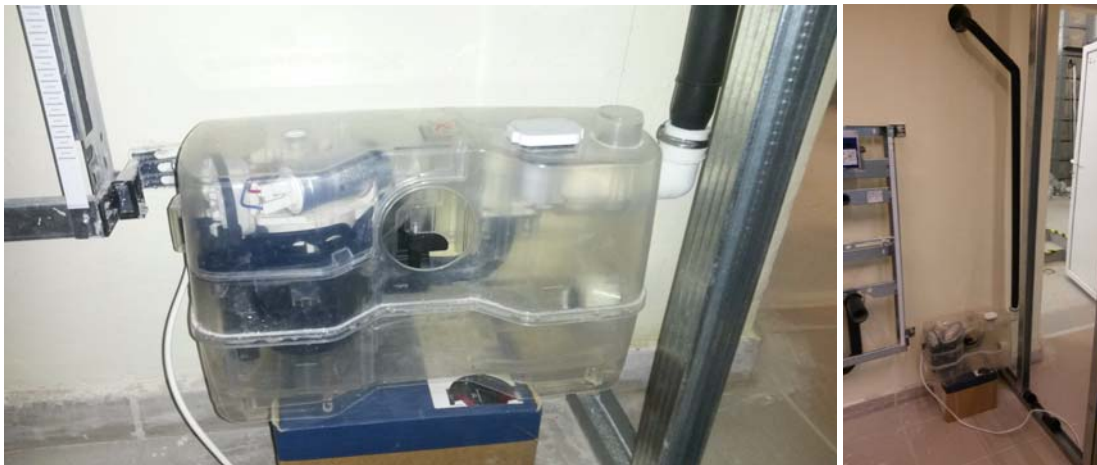
Figure 4 Pump ensuring the treatment plant inlet
