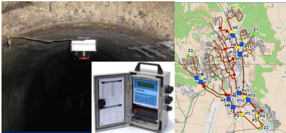
Figure 5 Water level meter placed in sewer system and its locations
