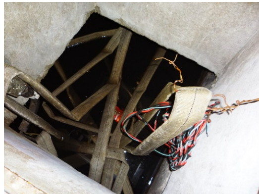
Figure 5 Inside the non-potable water reservoir
