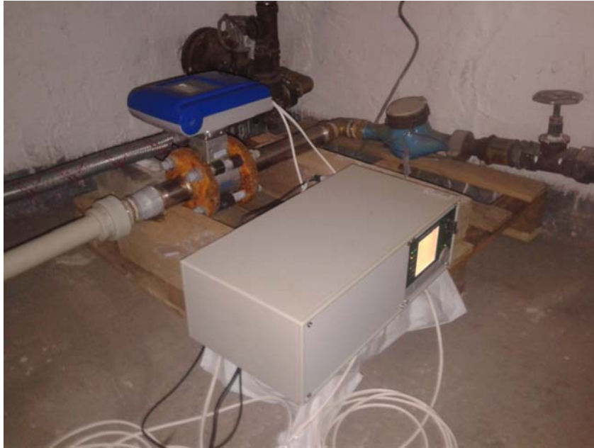
Figure 1 Data logger AHLBORN ALMEMO A 5690-2 TS, flow meter OPTIFLUX 1000 placed after water meter in residential building Ceskem Tesine
