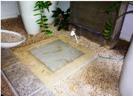
Figure 4 Access cover of the non-potable water reservoir
