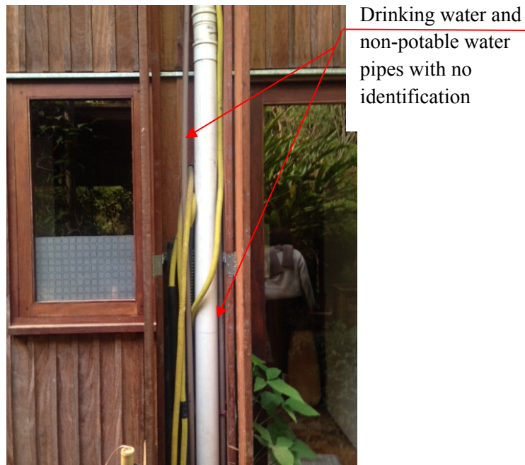
Figure 7 Inside a shaft with no identification that differentiates the pipe systems
