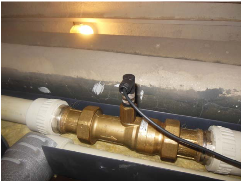
Figure 2 Flow meter VT 4025 MSHNS000F placed on the main supply pipeline of hot water in residential building Brno
