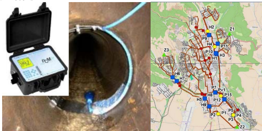
Figure 4 Flow meter placed in sewer system and its locations
