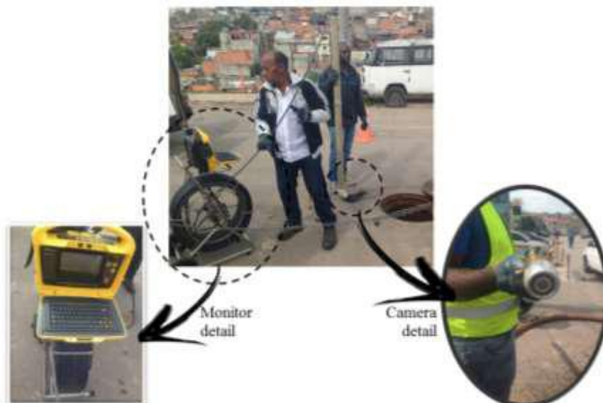
Figure 11 System used for the real time video of the sewage system pipe
