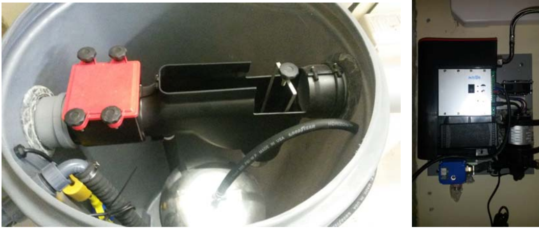
Figure 6 Submerged MBR, bioreactor with the filter for mechanical particles and pump supplying system with white water
