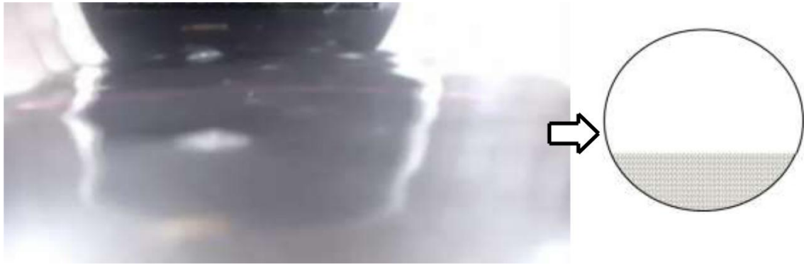
Figure 18 Solids accumulation near the Manhole n°2
