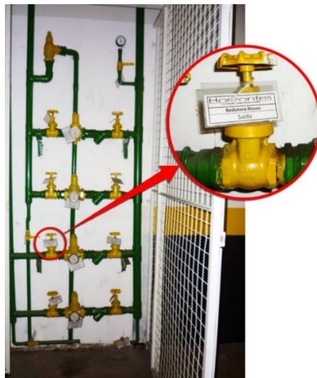
Figure 3 Pressure reducing station of non-potable water with the same color as that of the drinking water pipes
