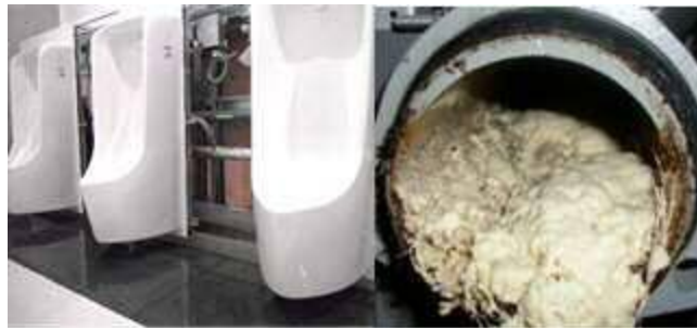
Photo 1 Horizontal branch drainpipe for urinals and appearance of adhesion and deposition of calcified urine in the drainpipes
