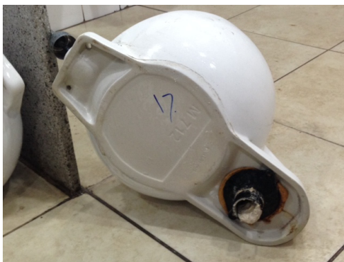
Figure 2 - Urinal removed during maintenance
