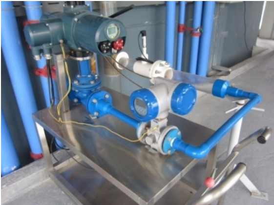
Fig . 6 Steady flow drainage equipment
