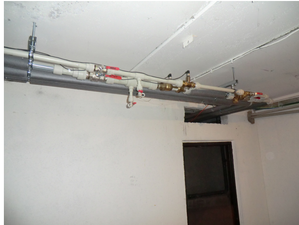
Figure 3 - Location of flow meters in dormitories
