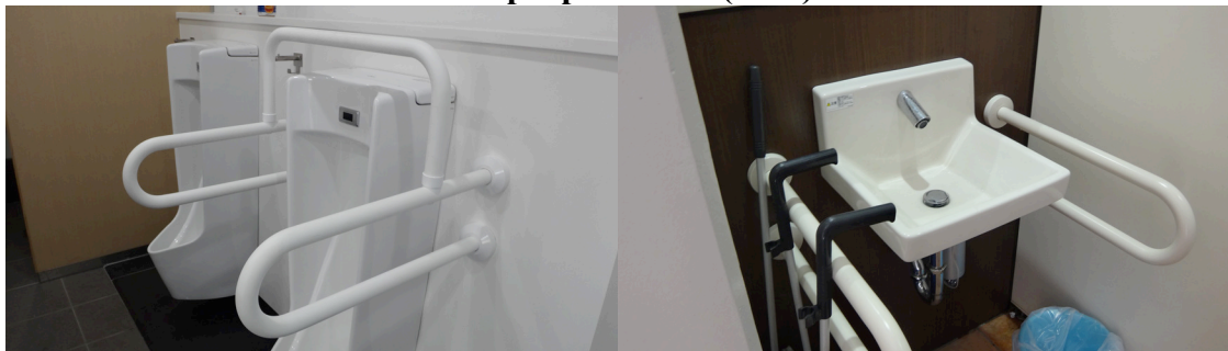
Handrail for handicapped person (left: No.A, right: Kawagoe station west)
