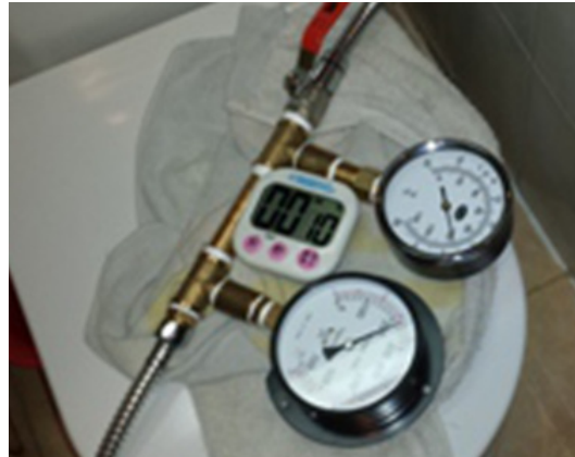
Figure 1 - Pressure and temperature gauge
