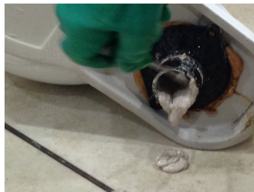
Figure 3 - Detail for the pasty material removed from the urinal during maintenance
