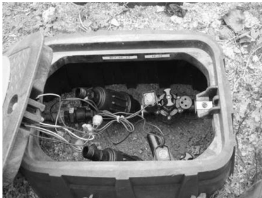
Figure-22 Solar powered soleriod valve-solenoid valve inside valve box
