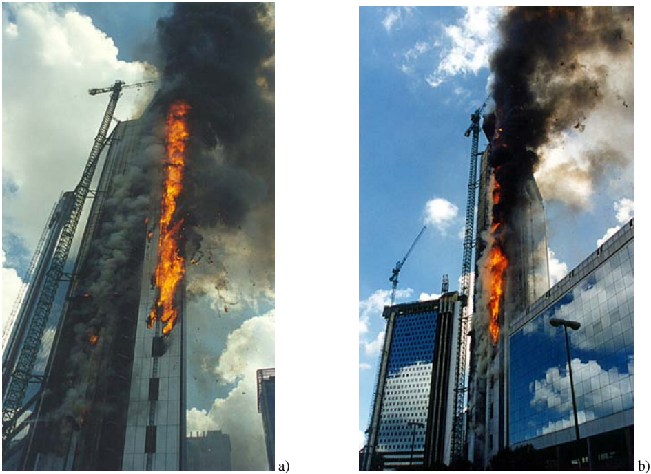
Fig. 1. a) The fire in high-rise building construction. b) The fire involved ACP panels
