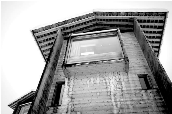
Fig.3. Current condition of the façade, Leis Unterhus
