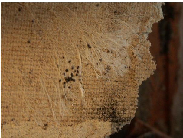
Pic. 3 Distinctive fungus mycelium at the back side of a gypsum board layer of a sandwich insulation board of polystyrene and gypsum board (DFWZ QLB)
