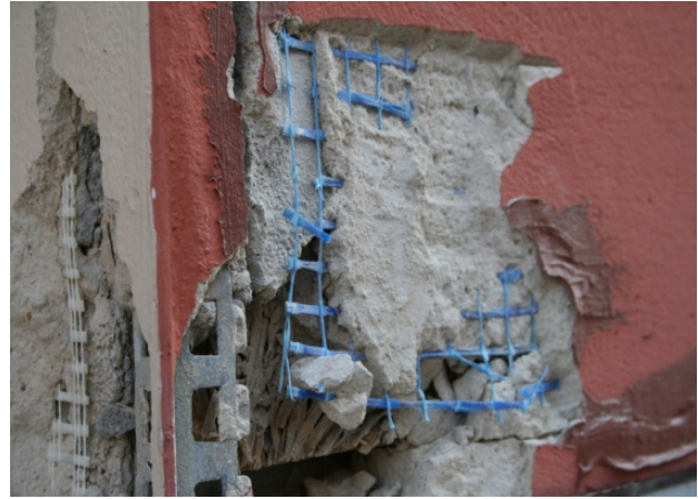
Pic. 4 Performance deficiency: The fabric insert in the plaster coating ends approximately 2 cm before the external corner and is not fixed around it. The corner profile is not conform to the system and has been fixed insufficiently on the subsurface. (DFWZ QLB)
