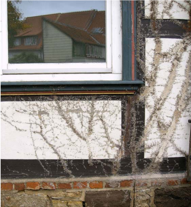
Fig. 5 Surface of infill and framework lumbers (coating and plastering) have been affected by anchoring roots of plants. (DFWZ QLB)
