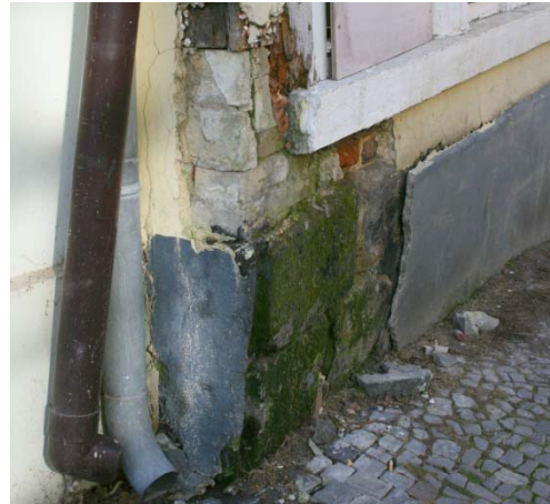
Fig. 2 The cement plaster discoidal scales off from the sandstone. Additionally, the moisture load was forced by defective roof drainage, so that in the sill plates and in vertical pillars timber-destroying fungi could spread. The sandstones are grown over by algae and moss. (DFWZ)
