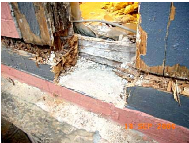
Pic. 1 Excavated wall construction, clearly visible is the extremely damage of the sill plates and the rising upright caused by brown and white pocket rot. The glass fibre-glass-insulation layer is viewable in the background. (private, wood preservation expert)
