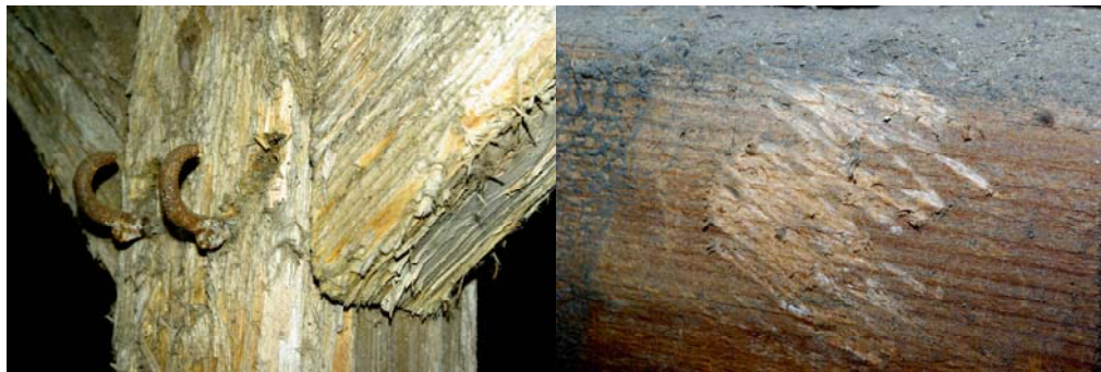
Photo 1 (left) Heavy corrosion
