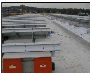
Roof surface with central row of light fittings and photovoltaic installation on the sides
