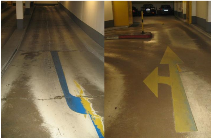
Image 1: Wear of surface protection systems in the range of ramps and curves in a car park
