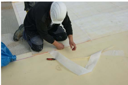
Figure 1: Application of a FBV mebrane on a blinding layer before reinforcing and concreting [source: DBV, Kiltz]
